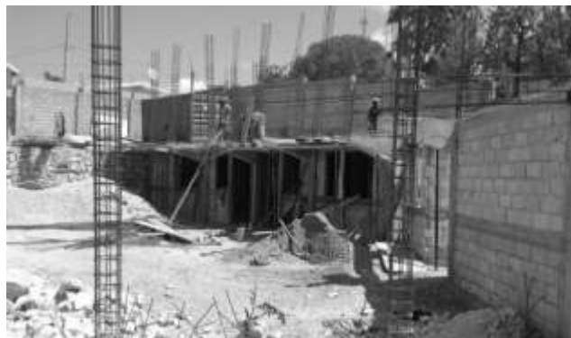
SOPUDEP is expanding! A second school building is under construction, largely by volunteers.
